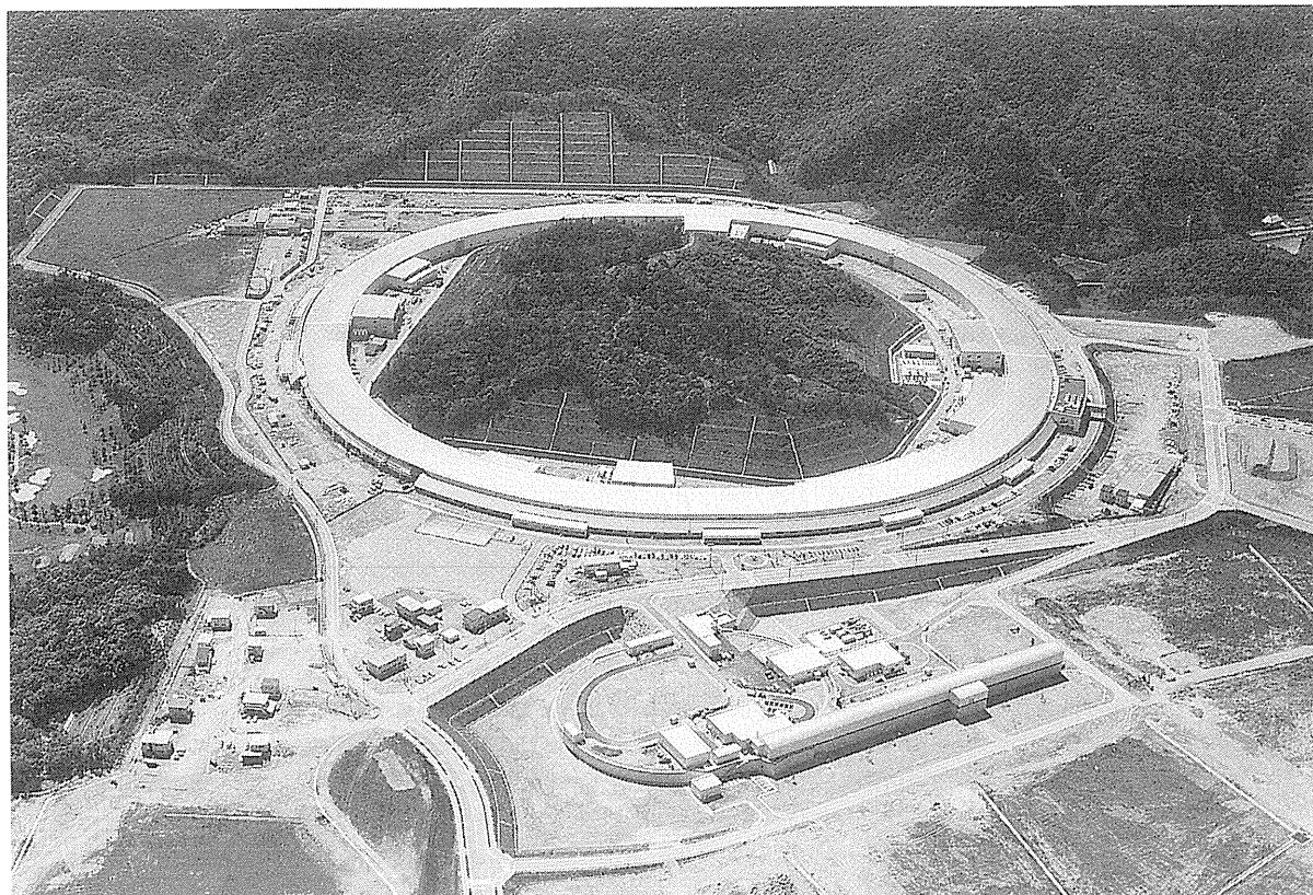
Figure 1. A bird's-eye view of the SPring-8 facility. The facility is under construction.
